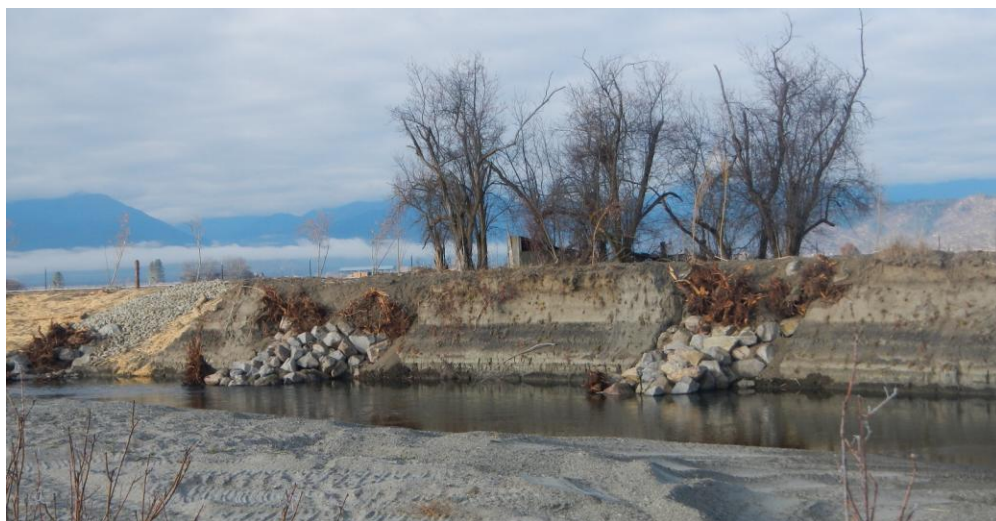
Photo 5: Downstream end of completed bank stabilization at River Mile 36, November 2013 (Siskiyou RCD).
