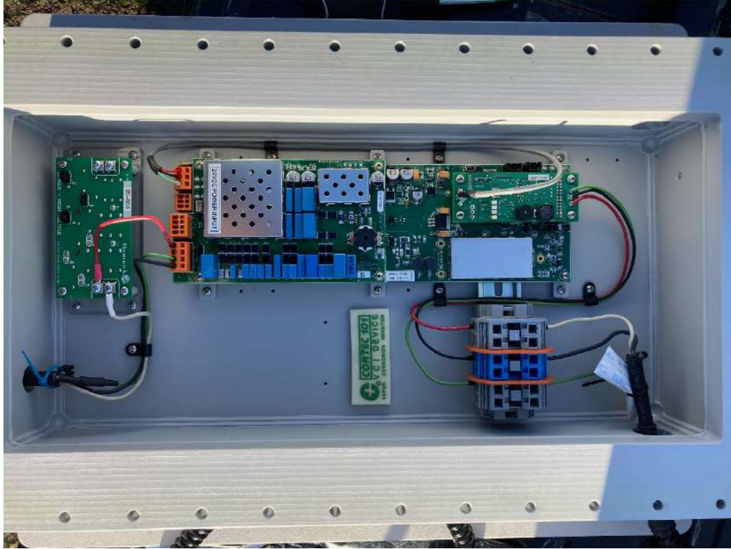
Picture 3. Fishway enclosure housing IS1001 reader and capacitance board.
