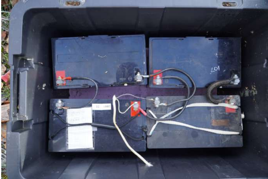
Picture 9. Example of battery bank setup at array site.
