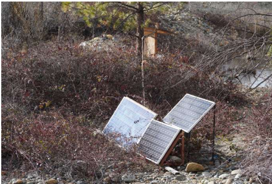
Picture 8. Example of solar panel setup at array site.
