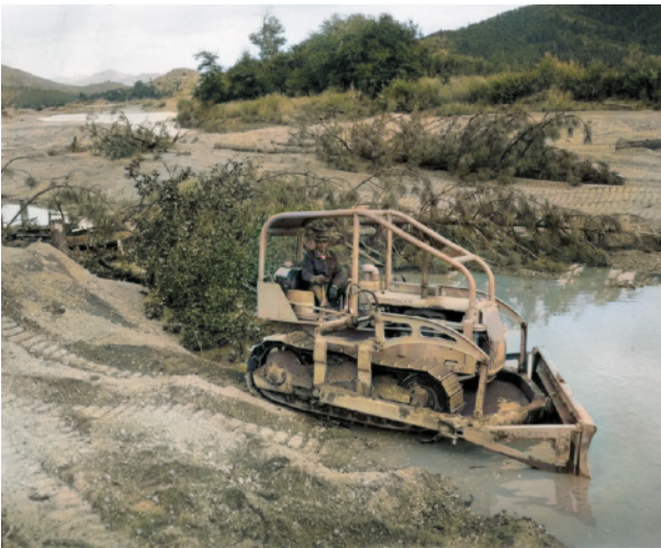
Lower Scott Valley Channel Stabilization. 1957. Tozier Brothers cabling trees to piling for jetties.
