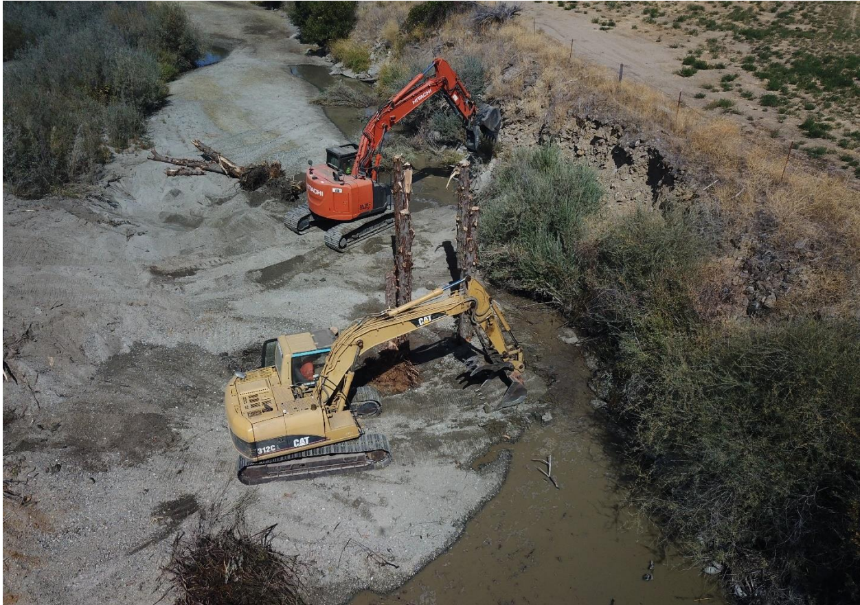
Construction of bio-engineered log jam on eastern bank of the Scott River, fall 2018
