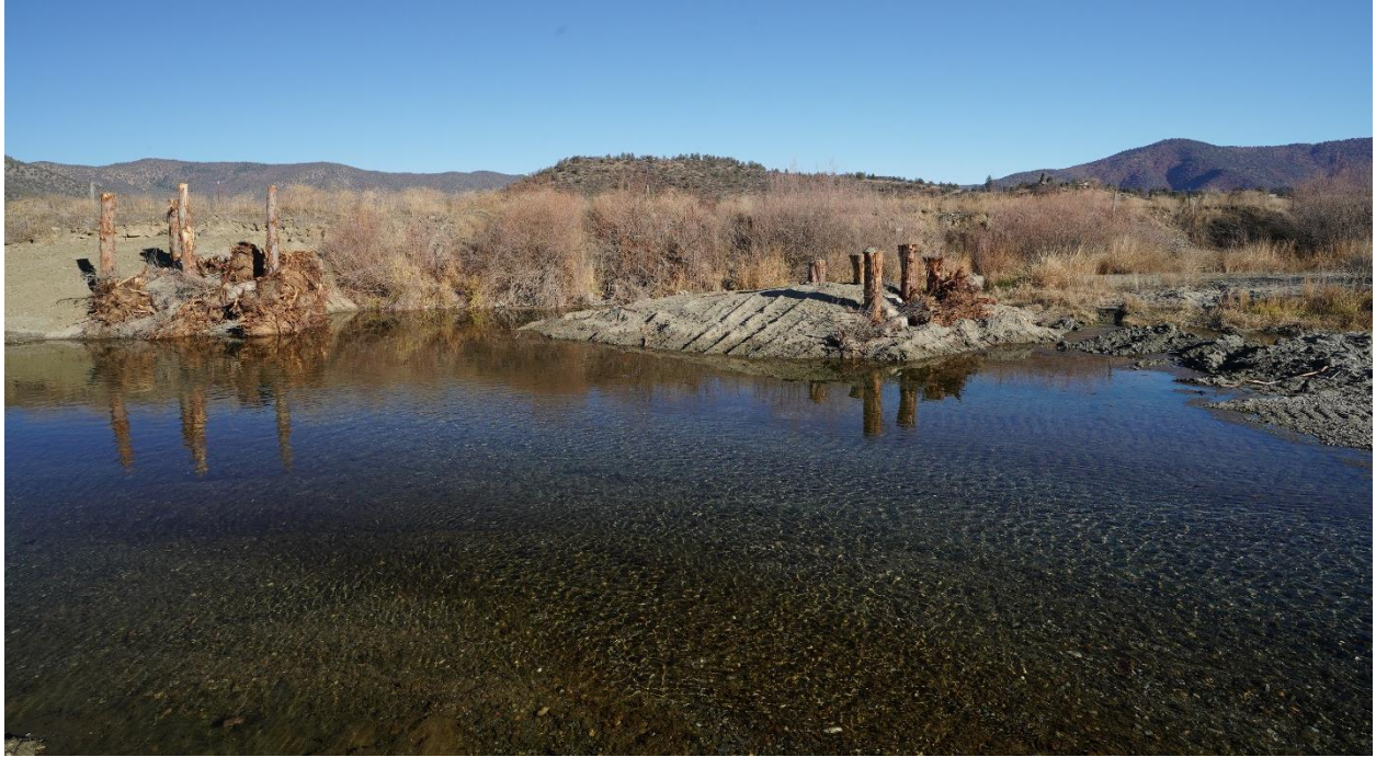
Figure 11. Type B ELJ (left) and Type A ELJ (right) after construction (eastern bank), 11/5/18.
