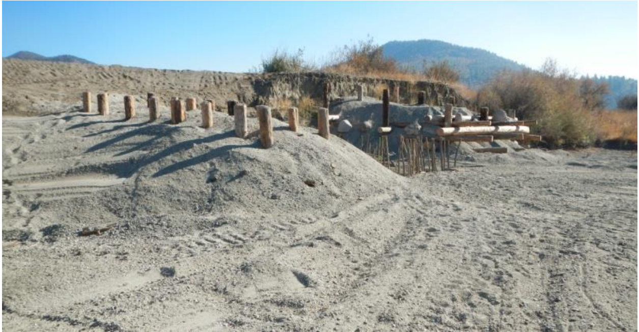
Figure 26. Type A ELJ (left) and Type B ELJ (right) after construction (eastern bank), 10/30/20.
