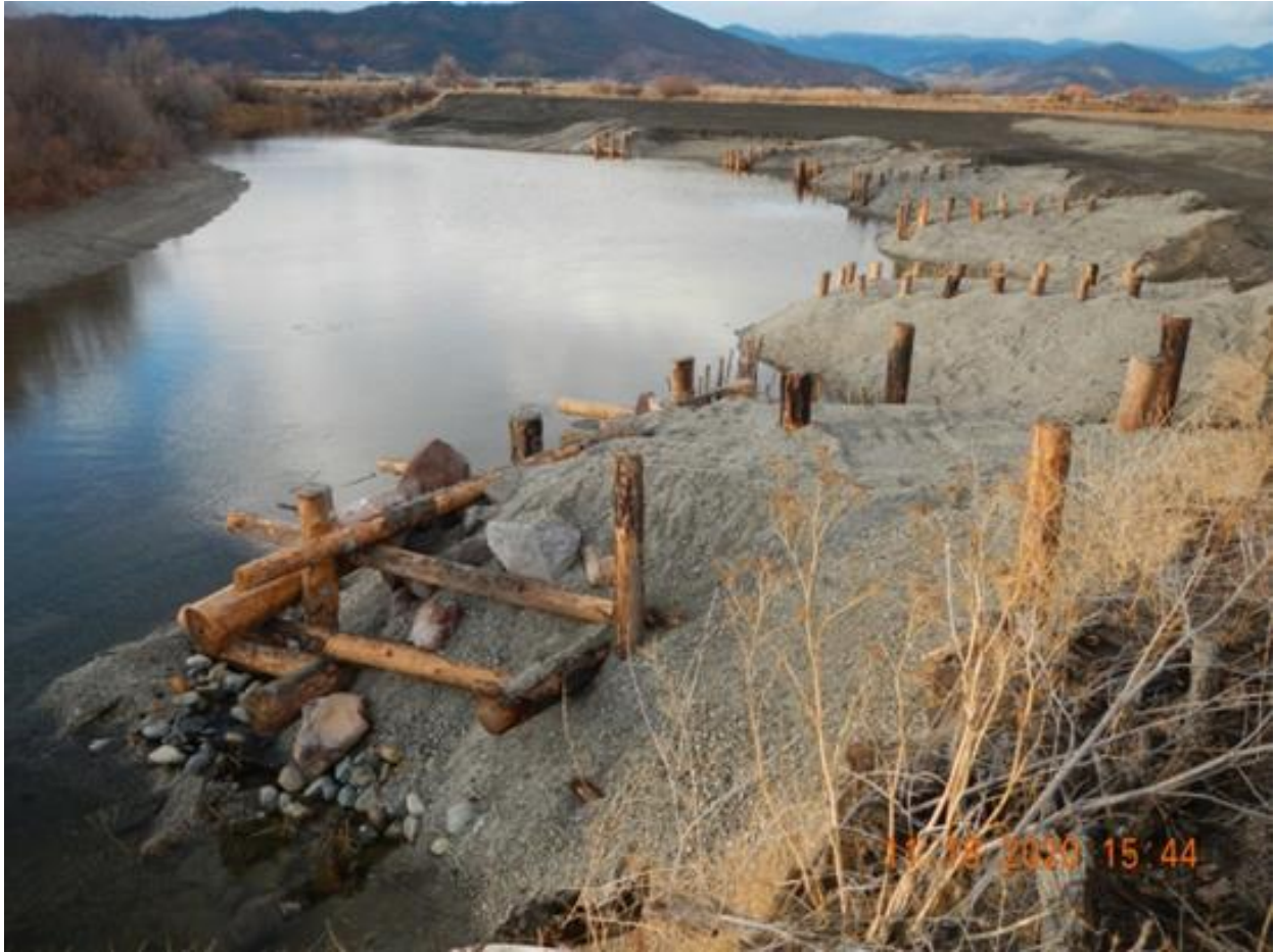
Figure 24. Type B ELJ (front) and all six Type A ELJs after construction (eastern bank), 11/18/20.
