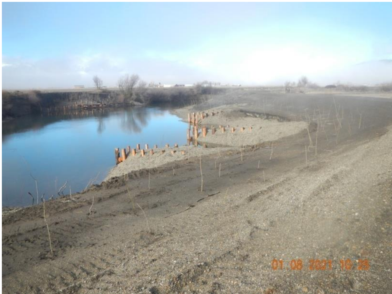
Figure 29. Willow poles and whips planted across the entire disturbed area of the eastern bank, 1/8/21.
